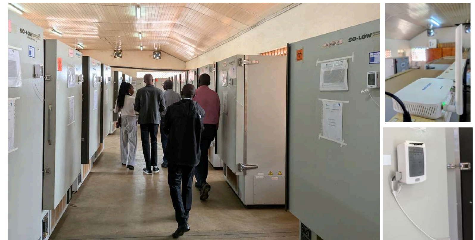
Inside the RHSP Kalisizo freezer house. On the right, the Dickson one temperature monitoring device.
