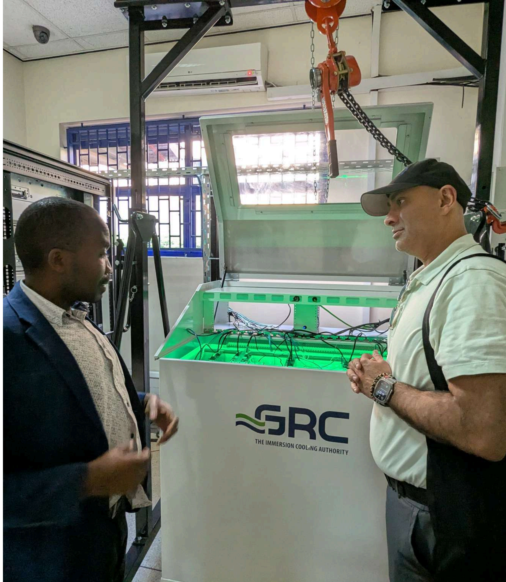
Ben Kakeeto, IT team member at RHSP taking Professor Akbar K. Waljee through cooling immersion system during the site visit at RHSP
